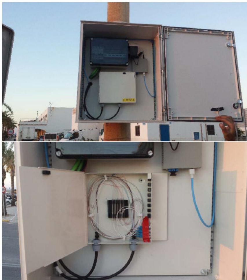
Detalle interior armarios báculos
